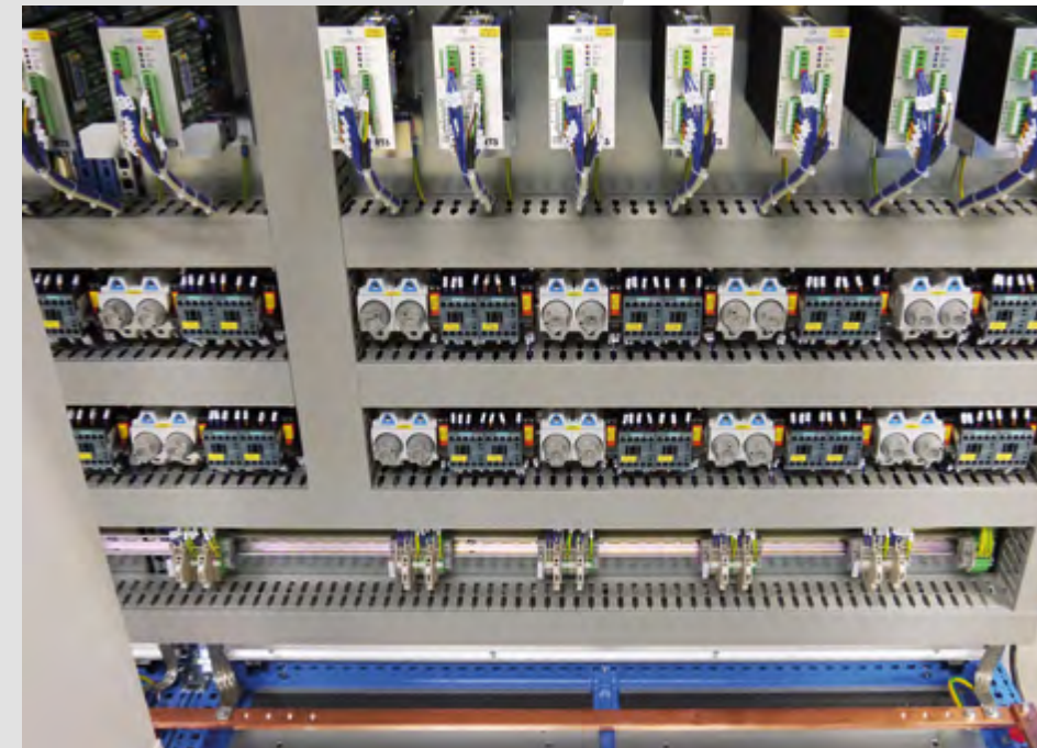
Retrofit at Lebbing: Making machinery fit for the future by installing the latest drive control system.
